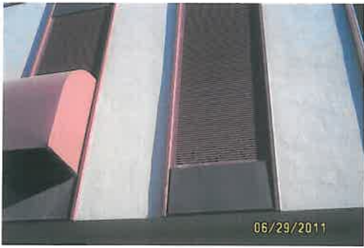
HVAC Unit NE Side, Outside air Intakes
