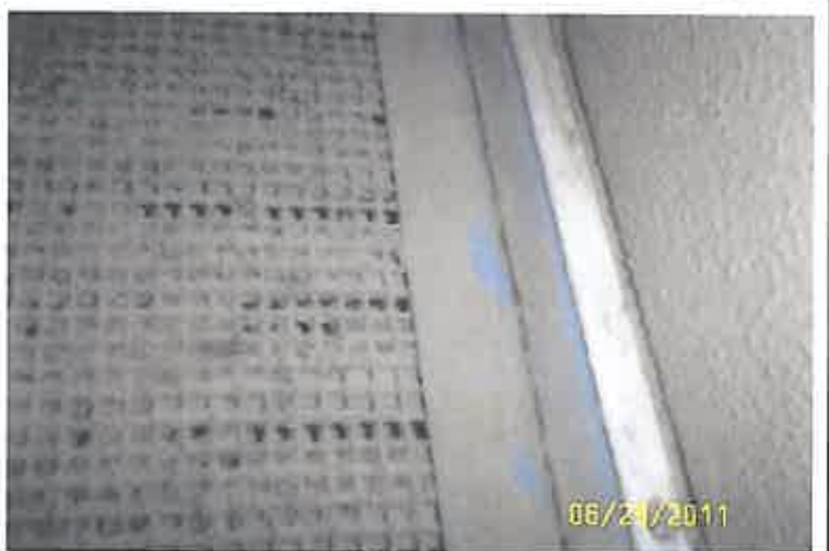
HVAC Unit NE Side, Same
