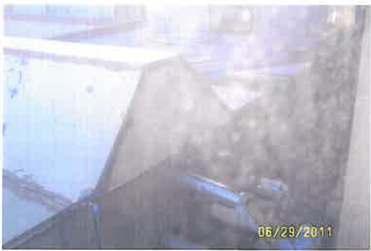
SSV Roof , HVAC unit Covered with Tarp to Prevent Rain from Leaking into Building
