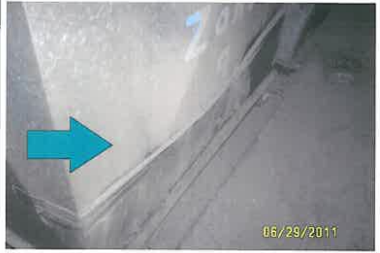
HVAC Unit NE Side, Shows how dust Accumulates on Duct from Air
