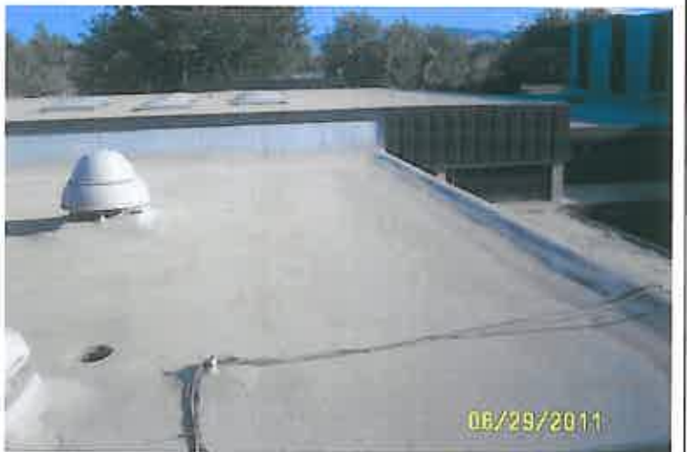
SSV Roof , Shows Accumulation of Desert Dust
