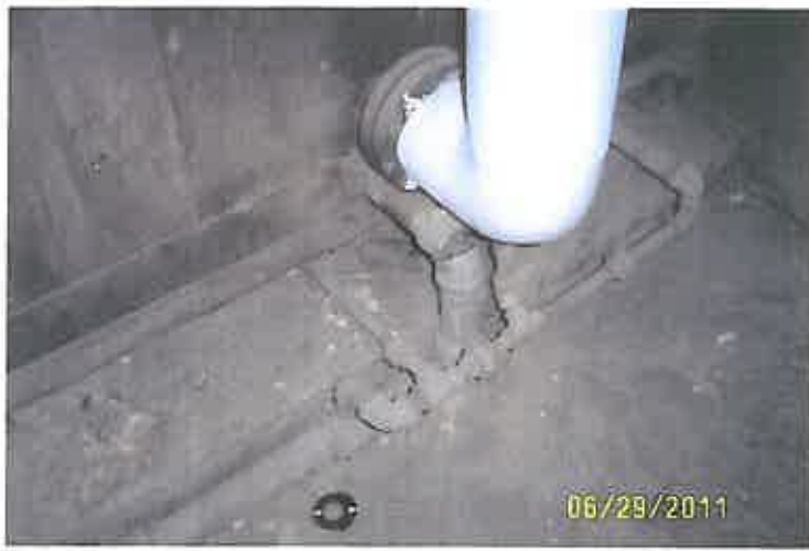
HVAC Unit NE Side, Debris on Floor
