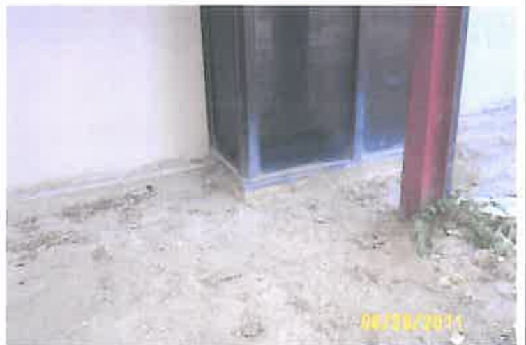
SSV Court Yard Some Excavation Done to Lower Grade so Water does not Enter the Building
