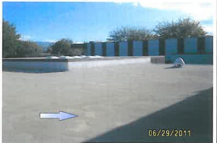
SSV Roof , Shows Accumulation of Desert Dust
