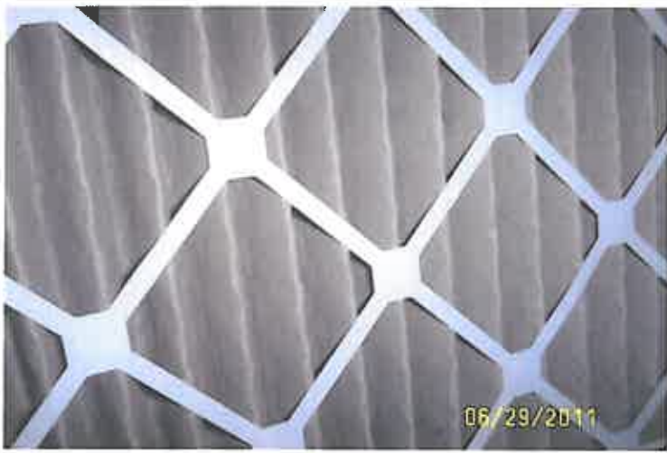
HVAC Unit NE Side, Build-up of Dust on Filters
