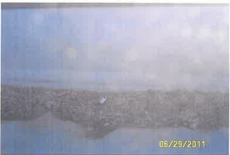
SSV Roof , Debris on Roof
