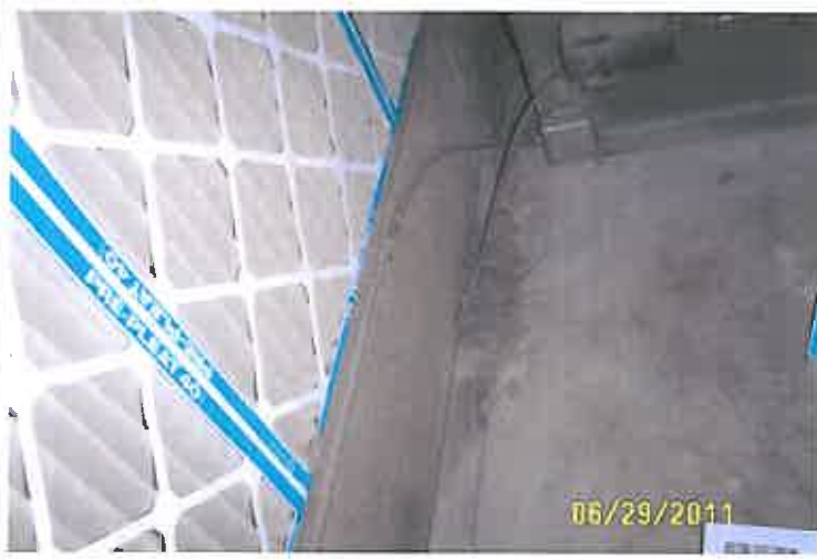
HVAC Unit NE Side Debris Inside
