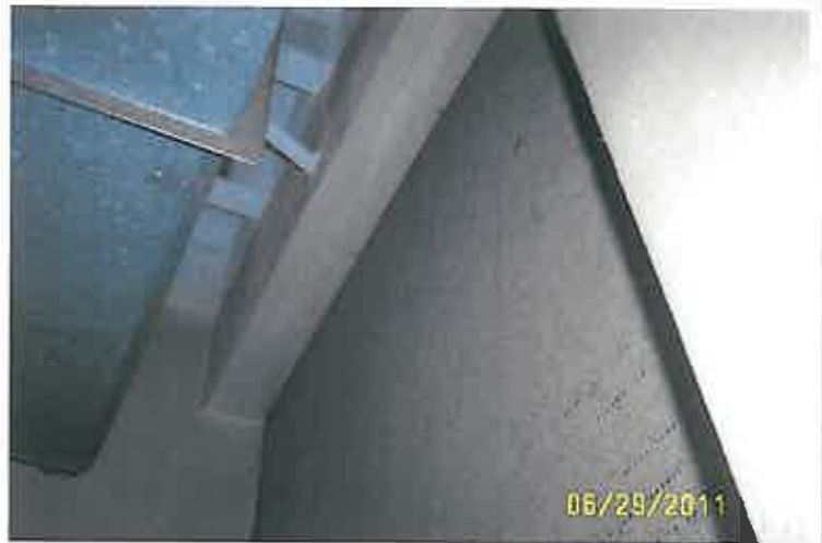
HVAC Unit NE Side, Same
