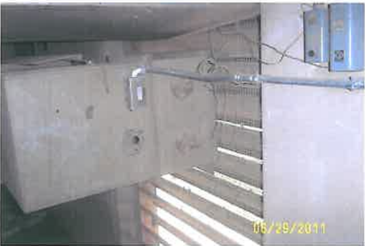
HVAC unit SW Side, Dust on Fresh Air Intake
