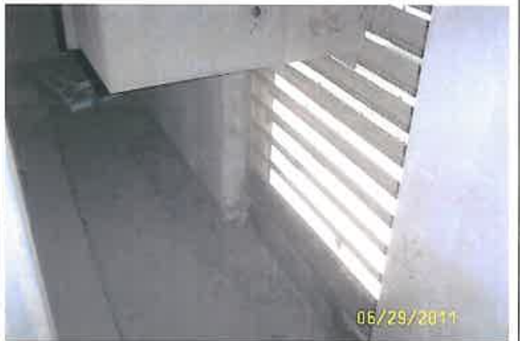
HVAC unit SW Side, Dust and Filters on Ground
