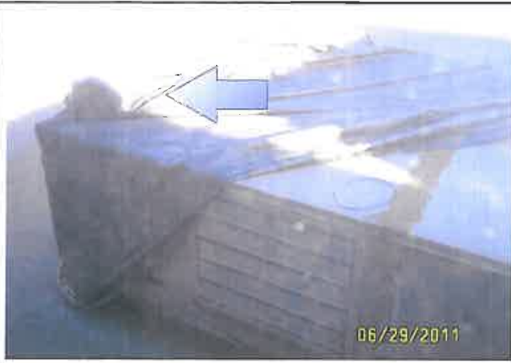
SSV Roof , HVAC unit Covered with Tarp to Prevent Rain from Leaking into Building, Motor Laying on Top
