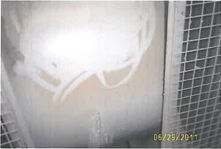
HVAC unit SW Side, Dust on Fan Housing
