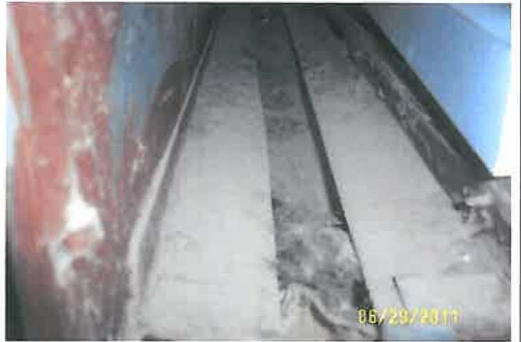
HVAC unit SW Side, Dust on top of Air Handler
