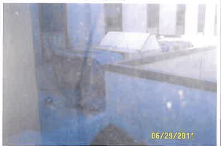
SSV Roof , HVAC unit Covered with Tarp to Prevent Rain from Leaking into Building
