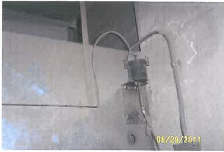
HVAC unit SW Side, Dust on Side of Air Intake
