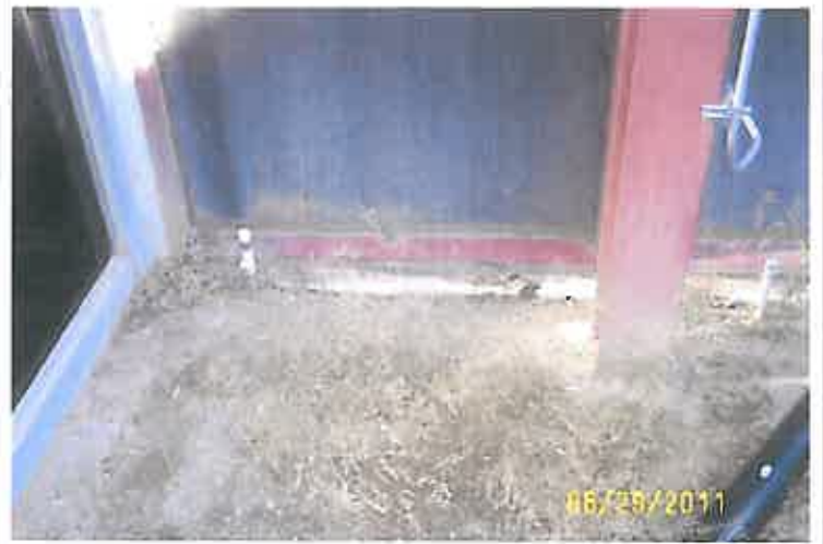
SSV Court Yard Water Damage to Exterior Window
