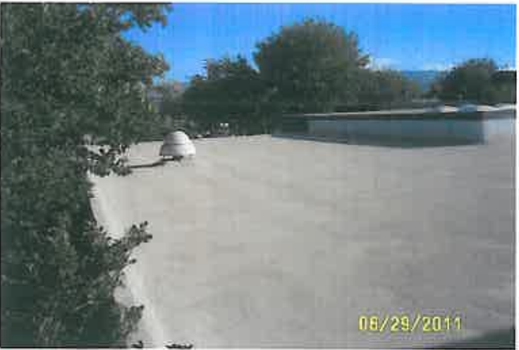
SSV Roof , Shows Accumulation of Desert Dust
