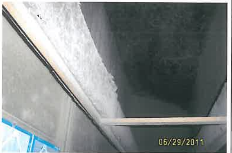
HVAC Unit NE Side, Fibrous Insulation in Side, Potential Source of Fibrous Material if more Duct is Lined with the Material
