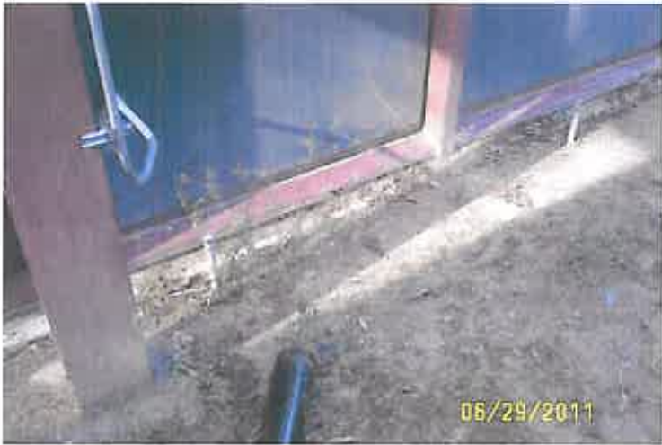
SSV Court Yard Exterior Window Rusted from Water
