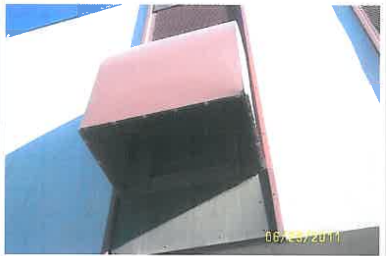
HVAC Unit NE Side, Same
