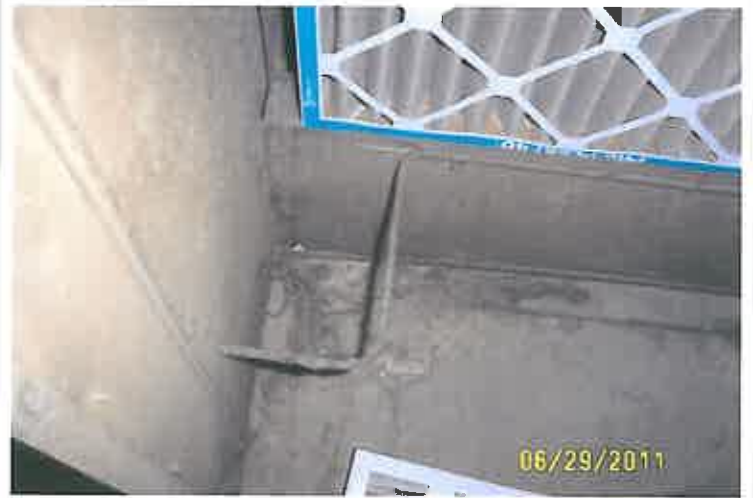
HVAC Unit NE Side, Debris Inside, Open Gap between Filter and Side of Unit, Filters Left Inside
