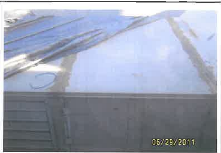
SSV Roof , HVAC unit Covered with Tarp to Prevent Rain from Leaking into Building
