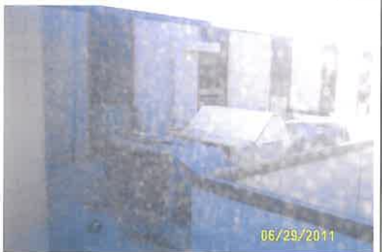
SSV Roof , HVAC unit Covered with Tarp to Prevent Rain from Leaking into Building
