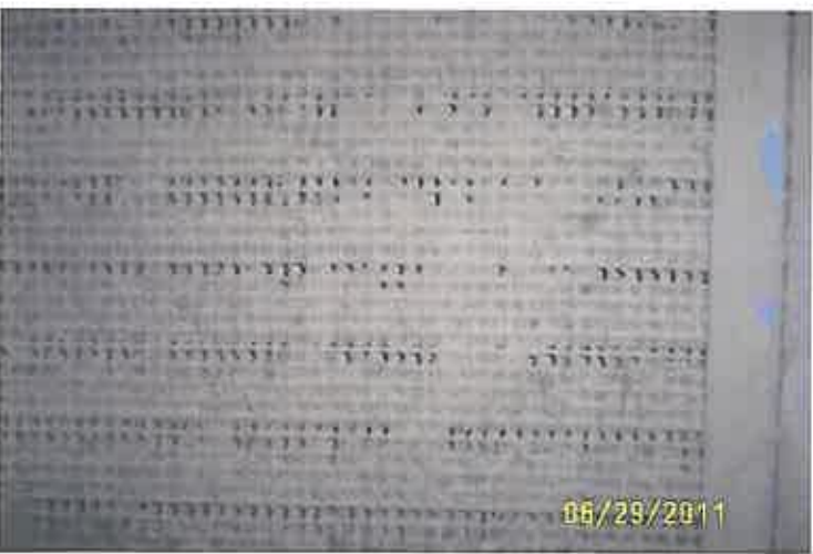
HVAC Unit NE Side, Same
